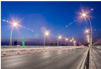
Road and Street Lighting
